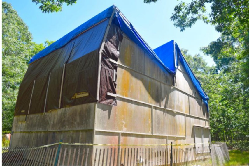
James Brooks's studio is in poor condition. Christopher Walsh
